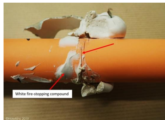
Cracking of a CPVC pipe due to incompatible fire-stopping compound – Hawkins, 2019
